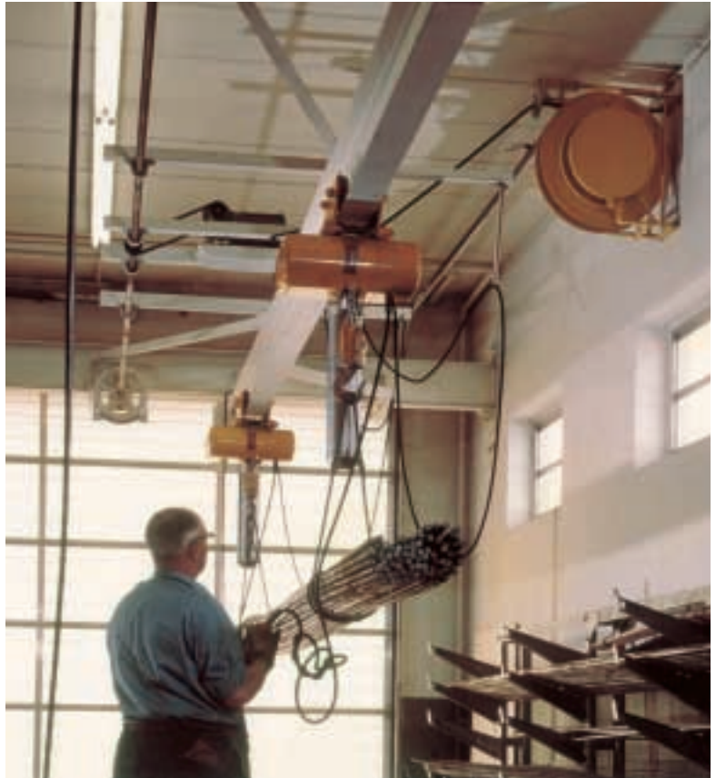
This Hannay cable reel mounted in an overhead installation provides electrical power to a crane in an industrial plant.
